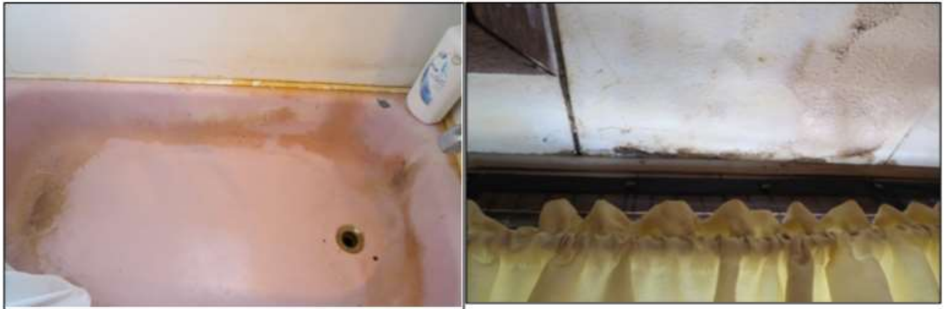
Image 3 and 4: Resident-provided pictures of water damage
